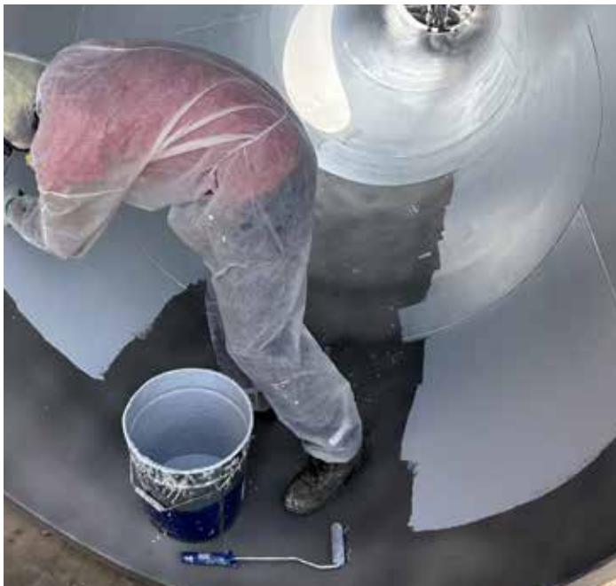
6. Primer Application - PENNGUARD™ HP Epoxy Primer being applied inside flue via paint roller
