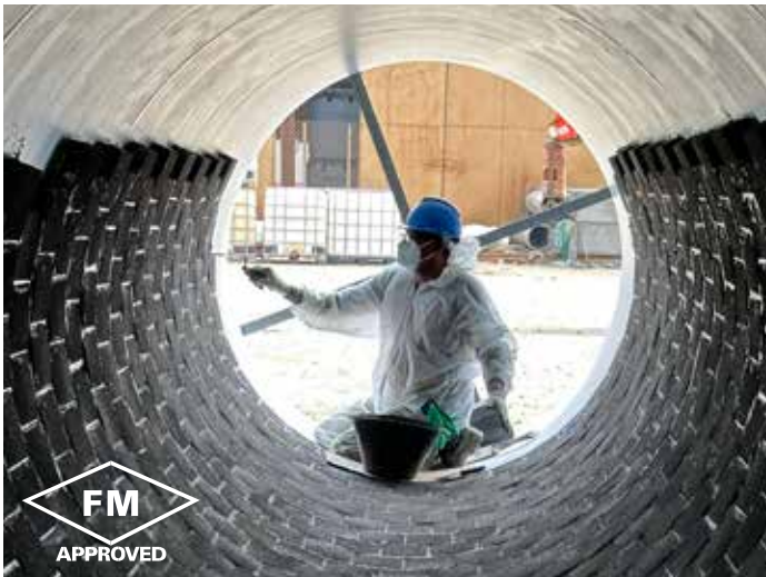
3. Small Diameter Flues - PENNGUARD Block Lining System being applied in a 1.7 m (5'7") diameter flue
