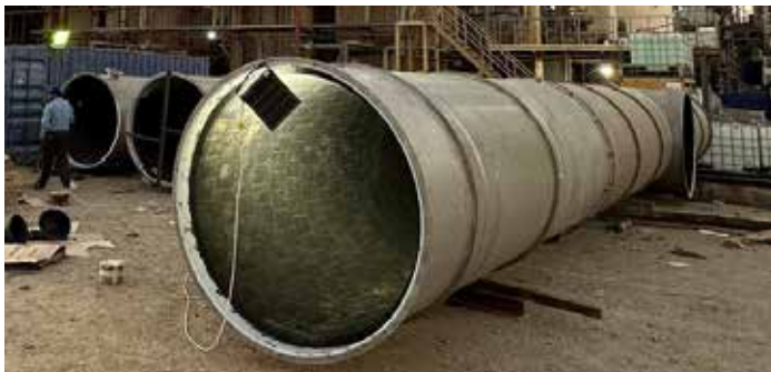
1. Project Laydown Area - PENNGUARD Block was applied to each section of a flue while laying horizontal on a ground level
