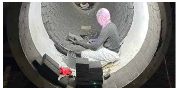
2. All day (24-Hour) Shifts - A flue being worked on at night using proper safety precautions
