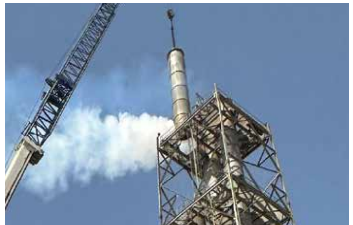
7. Flue Sections Craned Into Place - The gaps between the flues were then covered with PENNGUARD™ Adhesive Membrane and PENNGUARD™ Block prior to final inspection
