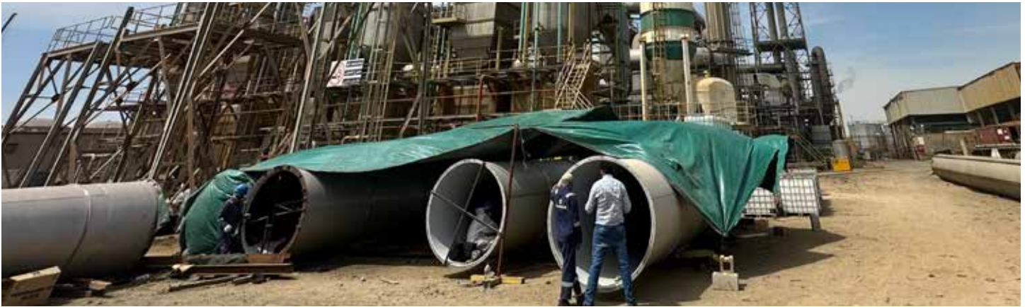
8. Job Site Perspective - The flue sections being coated in the laydown area were disassembled from the tower structure in the forefront
